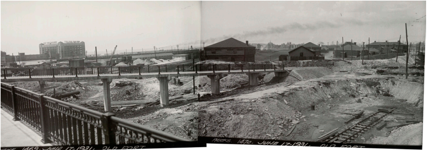
The new pedestrian bridge to the east gate of the fort on June 17, 1931, in two views by Toronto official photographer Arthur Goss. They are in a new exhibition in the Brick Magazine of photographs by Goss documenting work done at the fort during the 1930s. Source: City of Toronto Archives
